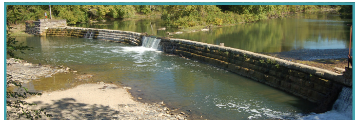
Water cascades through and over the deteriorating Thompson Mill Dam in Edinburgh in autumn 2023.
